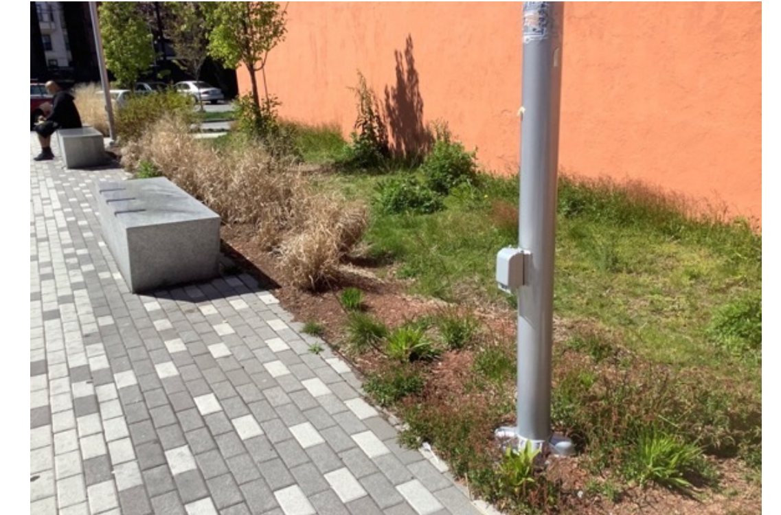
Electrical pole needs to be rewired
