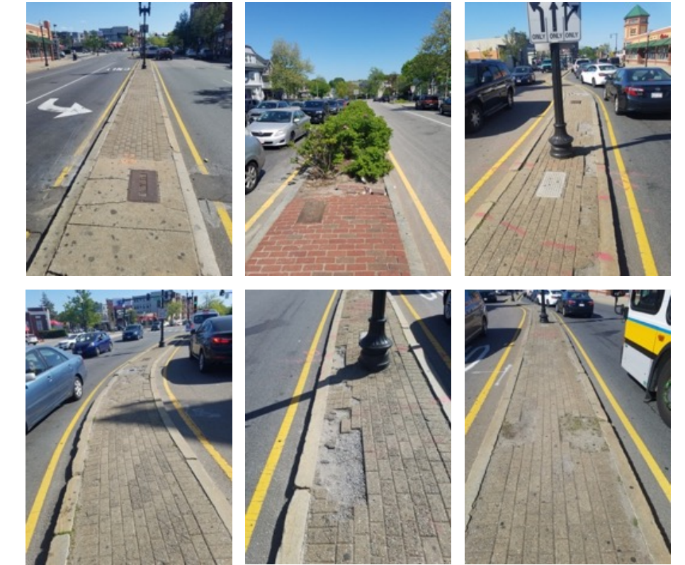
Cement median repairs needed
