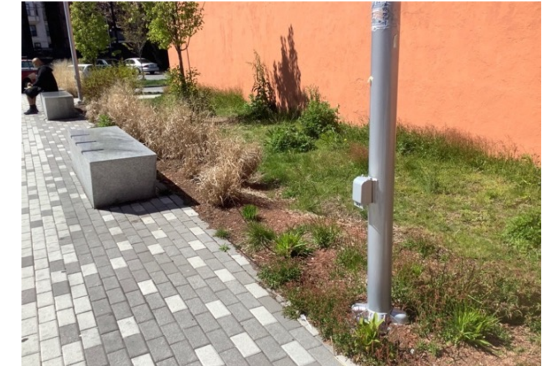
Electrical pole needs to be rewired
