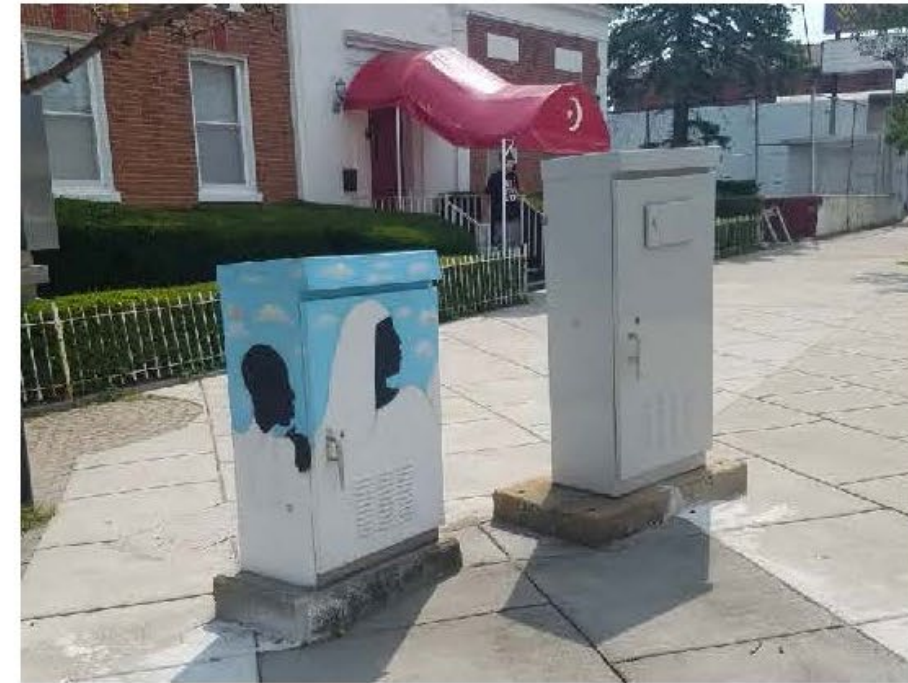
The bottom image shows the utility box where artwork needs to be repainted
