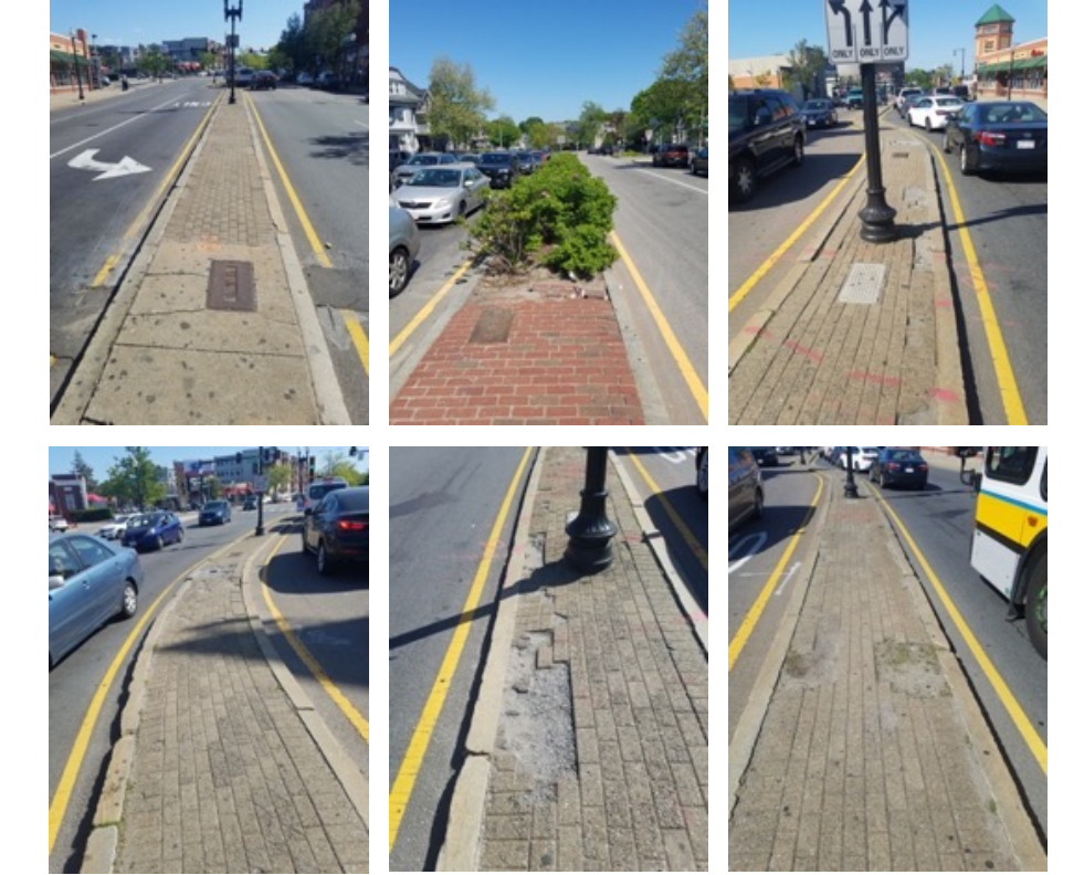
Cement median repairs needed
