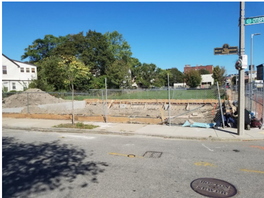
Thomas Construction has started work on a new laundrymat for the area.
